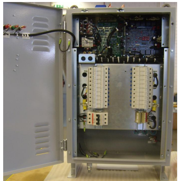
Internal view (dead front panel removed)
