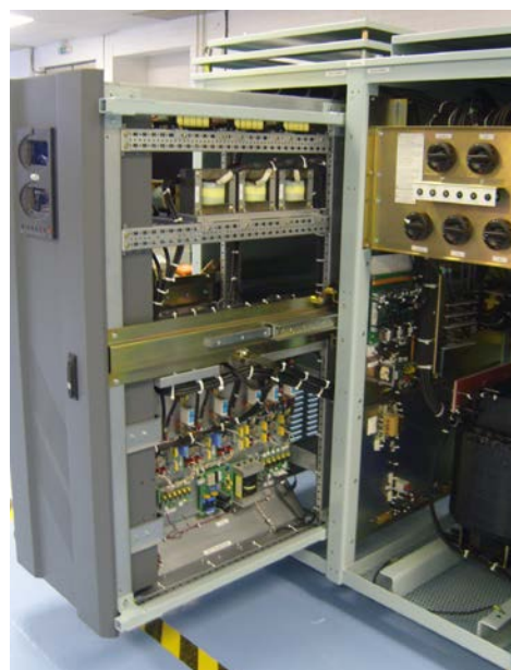
Internal view (power assembly withdrawn)
